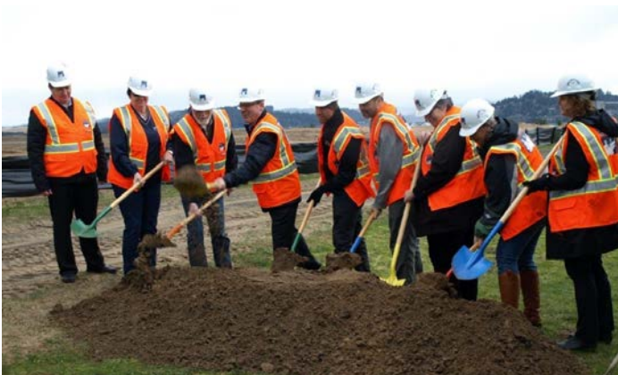
Ground Breaking— Future development of DHS— Department of Human Services, Child Welfare & Self Sufficiency Programs
